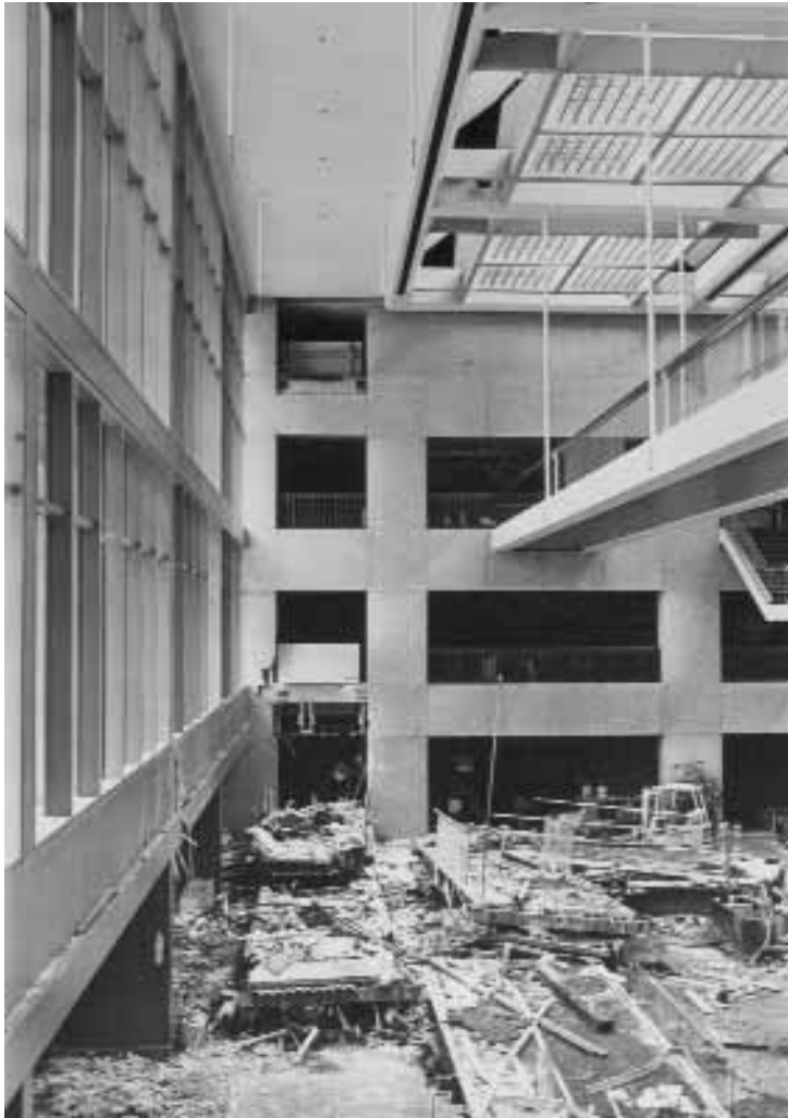
On July 19, 1981, the collapse of two bridges in the lobby of the Hyatt Regency in Kansas City, Missouri, resulted in the death of 114 people. The tragedy was the result of a construction change to the original hanger design.
